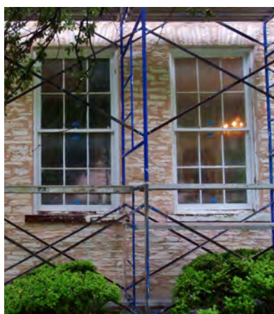
Scaffolding is installed on the north facade of the house for work on the windows.
