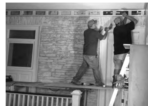
Original 18-inch thick limestone wall is stabilized by stairway to upstairs office as it connects to c1900 Cochran addition.
